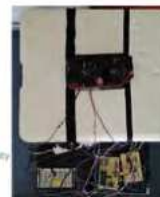
Fig.2: Picture of control room
