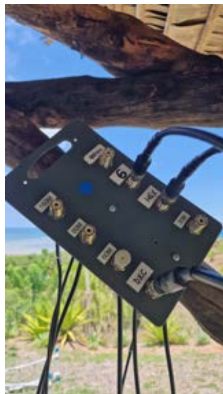
Coax patch panel
