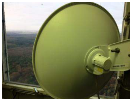
Powerbeam M5-400 Antenna 25dBi NOS site
