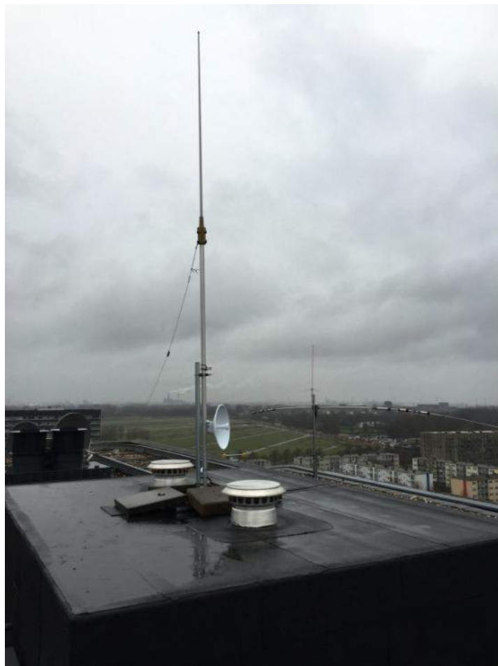
Vaste opstelling Powerbeam M5-400 Antenna 25dBi en Repeaters Amsterdam West site 1
